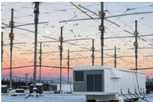
A section of the extensive HAARP antenna array and one of the transmitter shelters. [Photo courtesy of Jeff Dumps, KL4IU]
